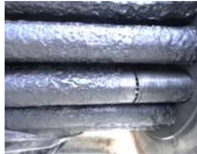
▷ Heavy Oil Screen filter
